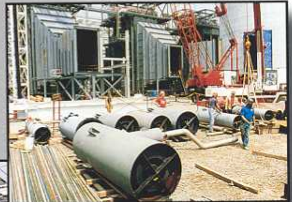
Steam Turbine Exhaust and Vent Silencing at Electrical Utility Plant
